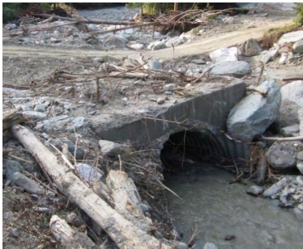
Severely Damaged Culvert, Stockbridge | Source: Chris Sargent
